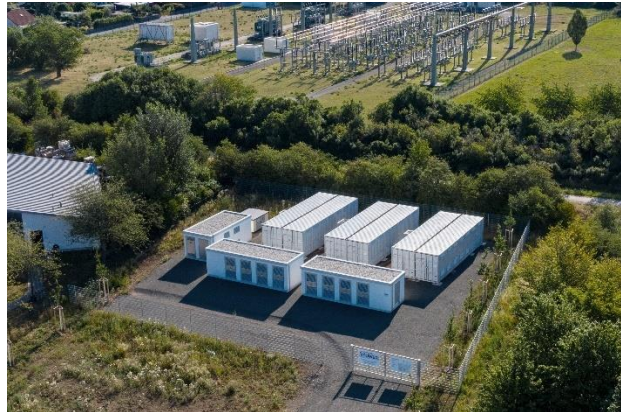
Diagram 6: Open space installation of a lithium ion mass storage system in container format
